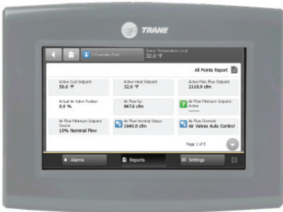
Figure 8 – TD7 operator interface
