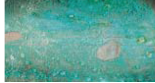
DEPOSIT CORROSION Deposits of algae and slime caused by inadequate water treatment.
