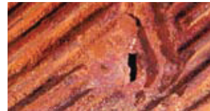
INTERNAL PITTING Caused by an abnormal presence of aggressive elements in water.
