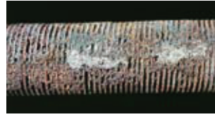
EXTERNAL CORROSION Caused by air intrusion.
