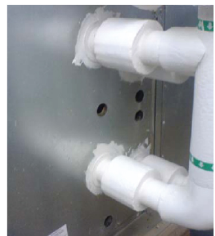
Figure 2. Unsealed coil drain and vent holes.
