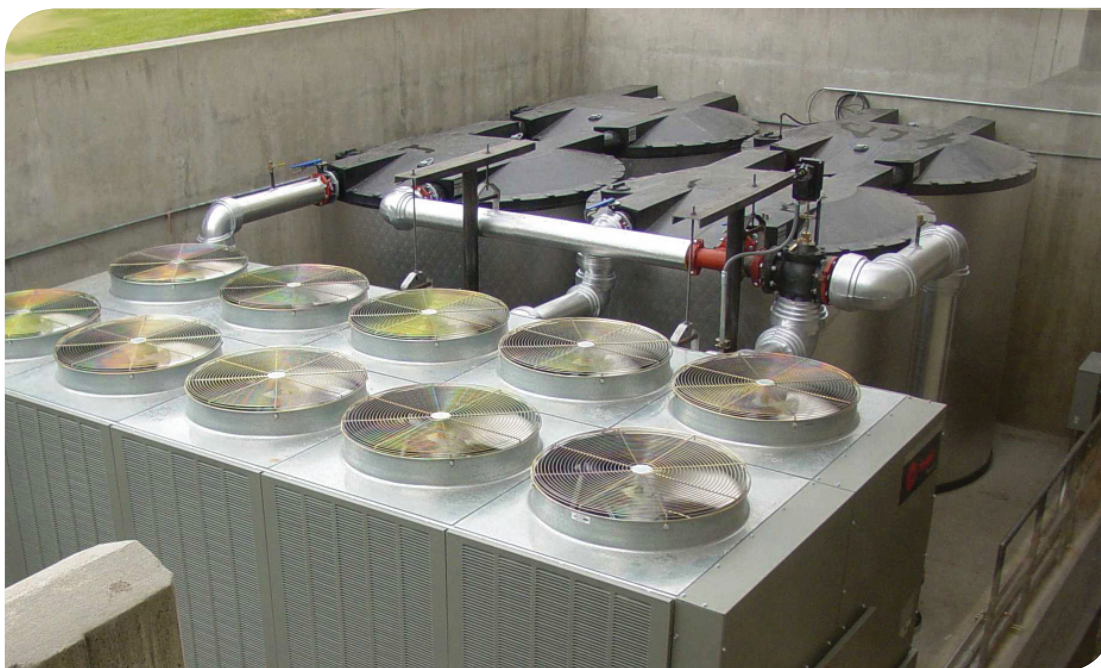
Four tanks occupy the space initially planned for a second chiller.
