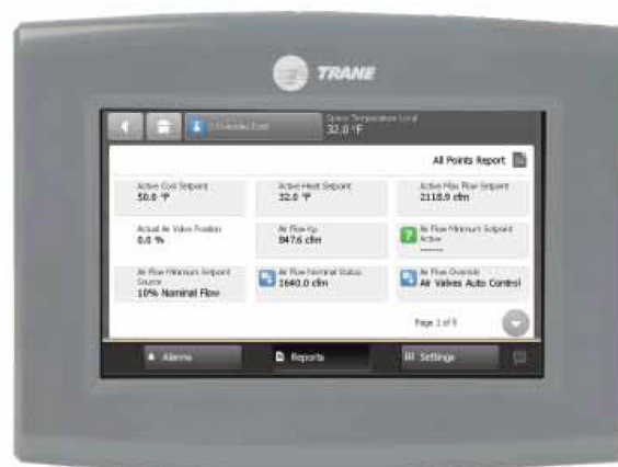
Figure 6 – TD7 operator interface
