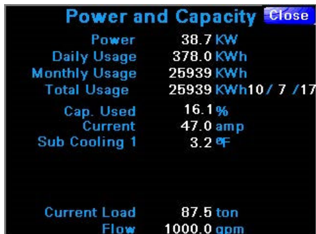
Figure 19. Power and capacity control screen
